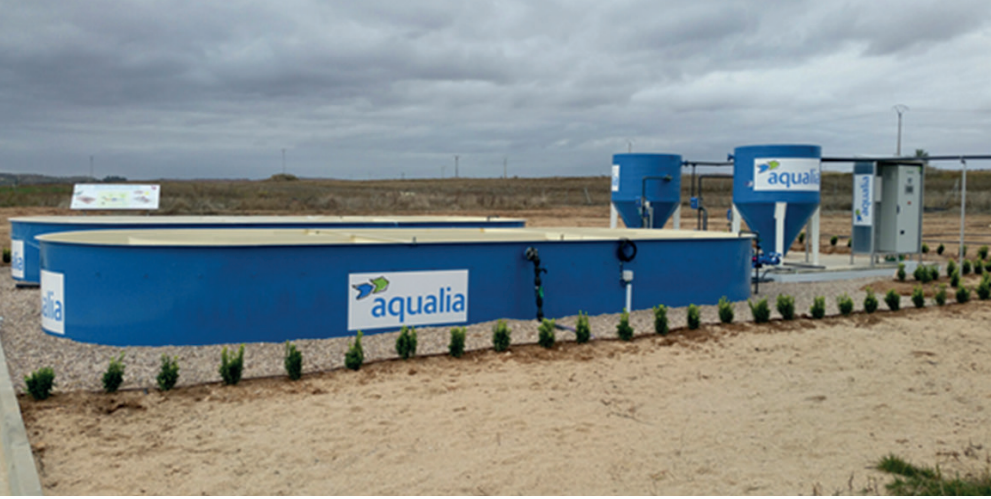
Demonstration treatment plant at the Estiviel treatment plant (Toledo).
